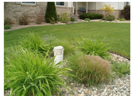
Attractive landscaping protects a 12-inch high wellhead.
